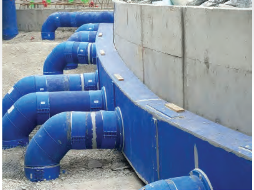
Continuous curved radius grill plenum was custom built to fit around the 100ft curved concrete wall shown here.
