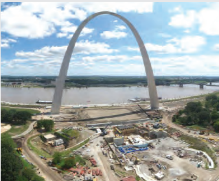
Installation of the The BlueDuct preinsulated The Duct System at the Jefferson Memorial Gateway Arch.
