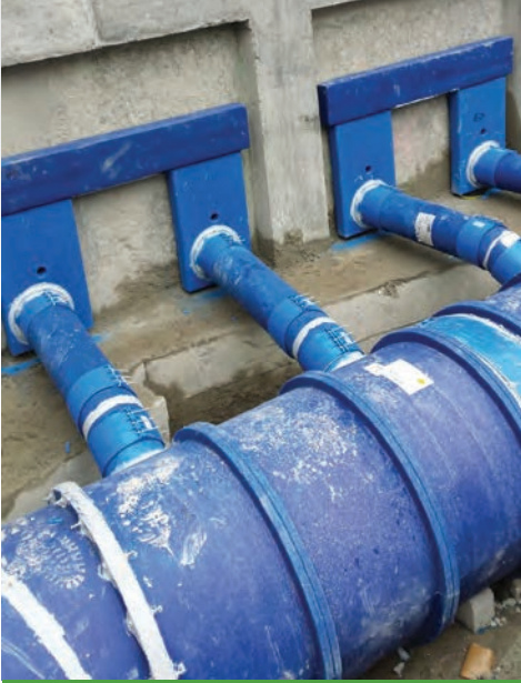
Diffuser boxes were mounted and ducted into the main trunk line after air testing was completed
