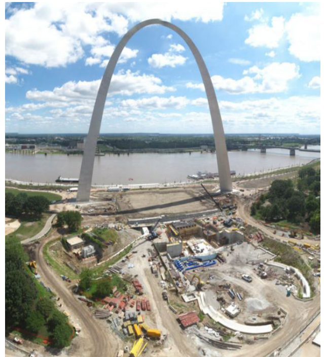
Installation of the The BlueDuct preinsulated Duct System at the Jefferson Memorial Gateway Arch.
